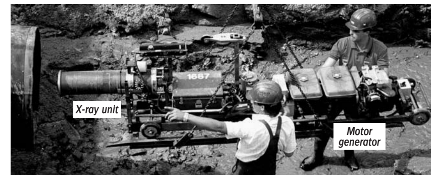
Fig. 12-18. Large diameter X-ray crawler with motor generator.
